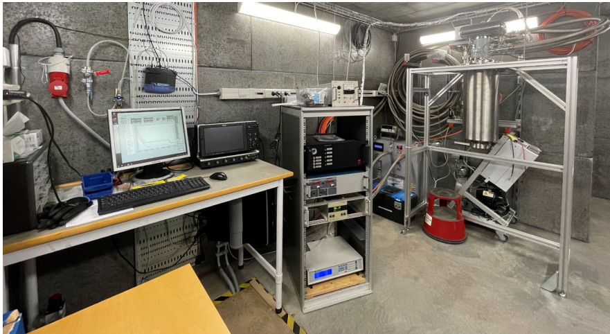
Fig. 1. Pulsed dc cryo system in a FREIA lab in Uppsala, Sweden
